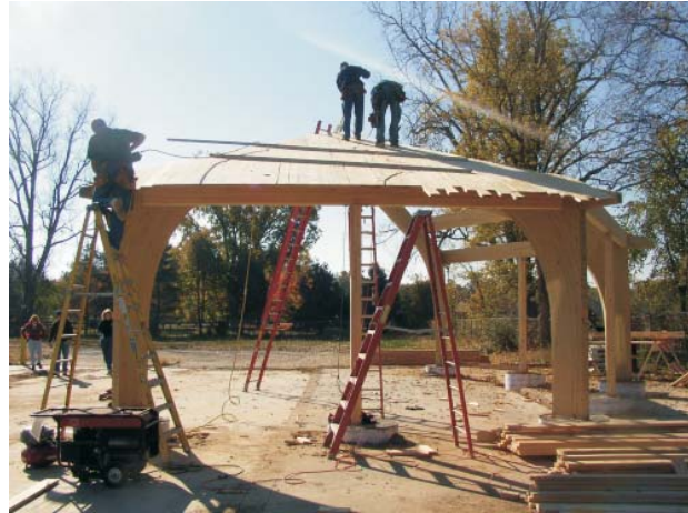
Rotarians construct band shell for the City along river walk for open air performances
